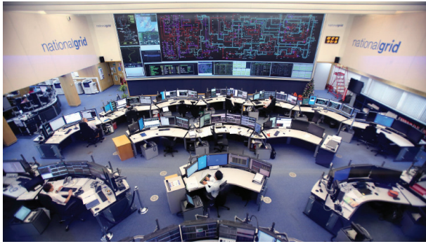
Figure 10. The United Kingdom National Grid control center. The United Kingdom's power flow is controlled and predicted here, with generators instructed to go online or offline depending on current national demand. Power can also be bought and sold from Norway and France. (Source: Financial Times UK)
